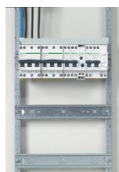
Installation Schneider Electric
